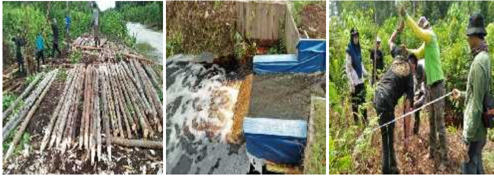
Picture 1: The Building of The Stuck Canal and The Monitor Well by Involving the Society Group of Lukun Village
